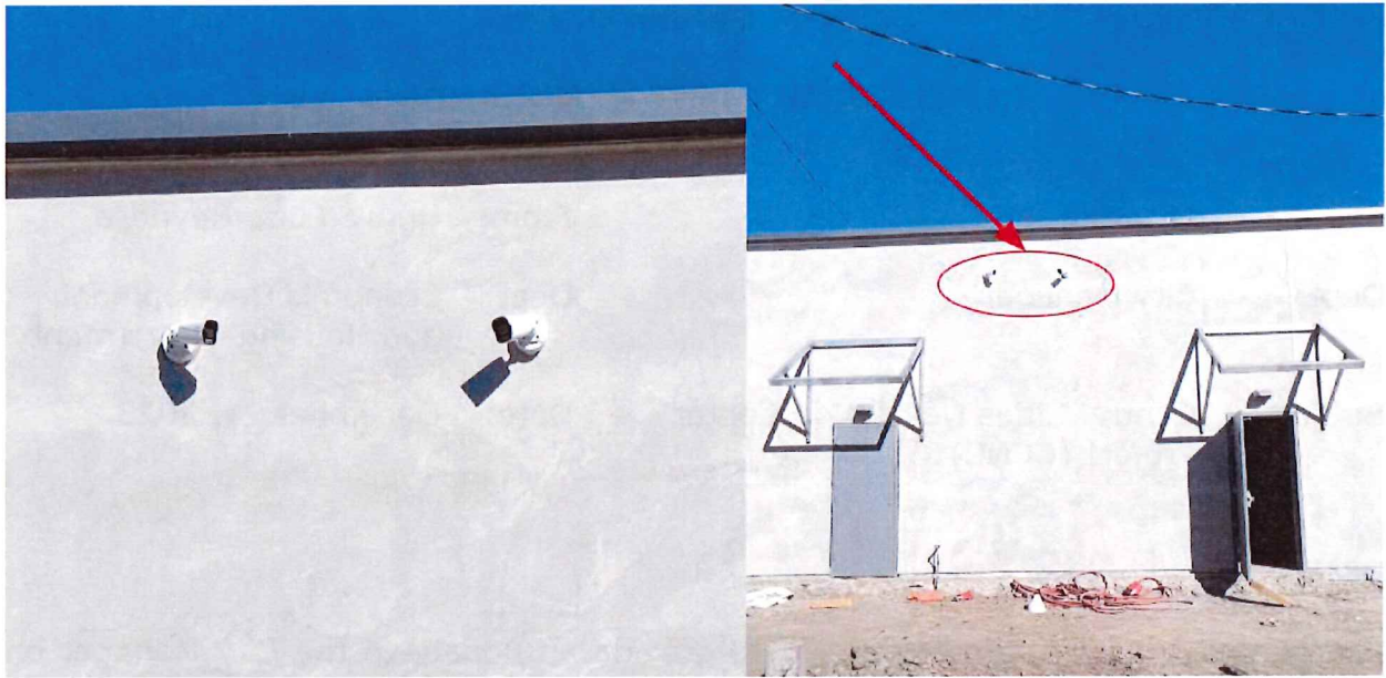
Photo: Security cameras installed
