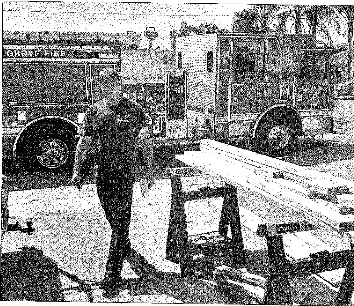
Courtesy photo Fire Engineer John Marquez and others from the Garden Grove Fire Department built a wheelchair ramp for a disabled resident in need last week.
